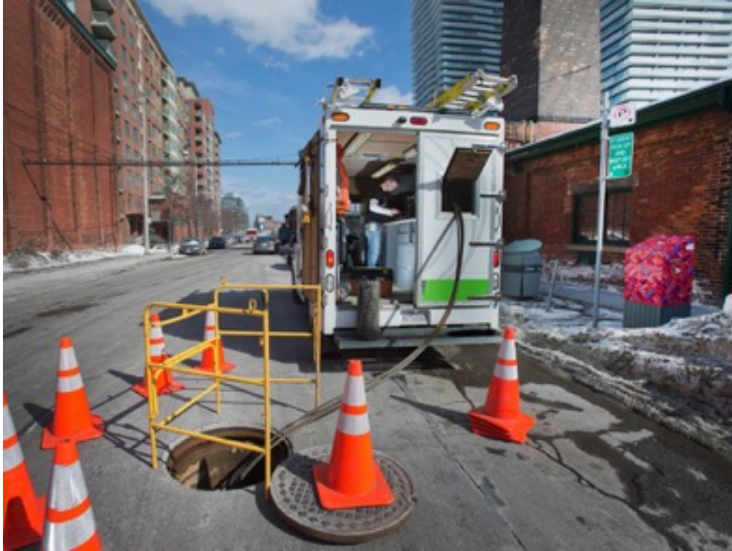
A Beanfield truck in the Distillery District, working to get the entire area connected to the ultra-high-speed service. Peter J. Thompson / National Post
